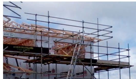
▲ Example of edge fall protection
